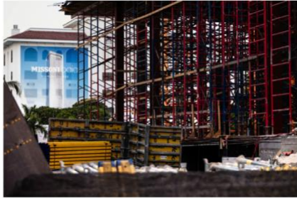
Missoni Baia, a 249-unit tower under construction in Miami's Edgewater neighborhood, in a licensing deal with the fashion brand Missoni. Scott McIntyre for The New York Times
